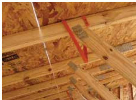
A pre-installed attic anchorage system.
